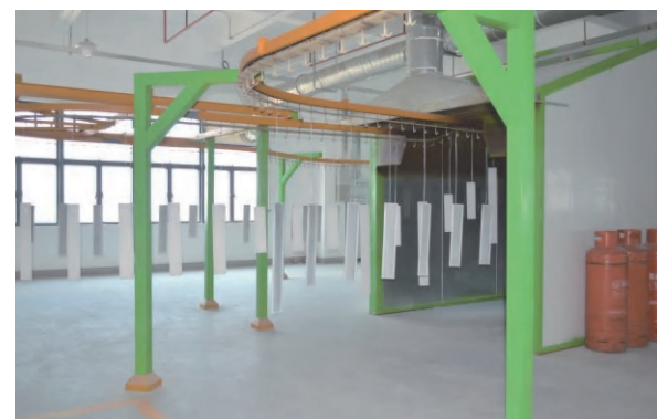
Spraying Processing Center
